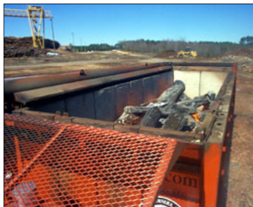
S-327 Firebox in Full Operation
