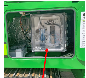
Emergency Transceiver Cable Storage
