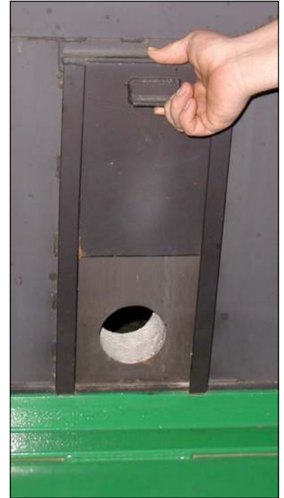
Access Door for Lighting
