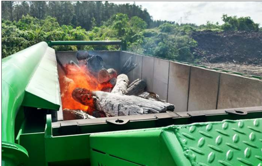
S327 FireBox in Operation
