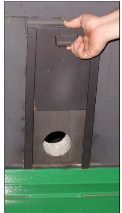
Access Door for Lighting
