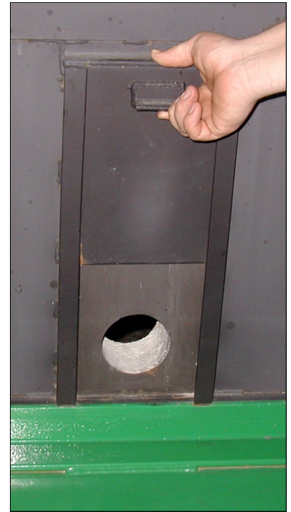
Access Door for Lighting
