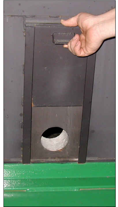
Access Door for Lighting
